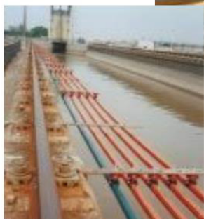
Water Treatment Works
