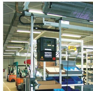
Fully integrated: A62 on an assembly line
