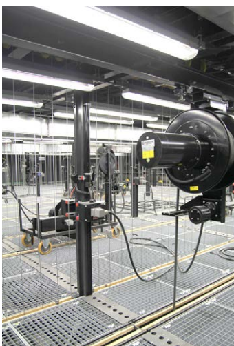
Slip ring assembly in theater (stage floor)
