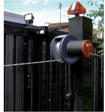
Slip ring assembly in gate locking system
